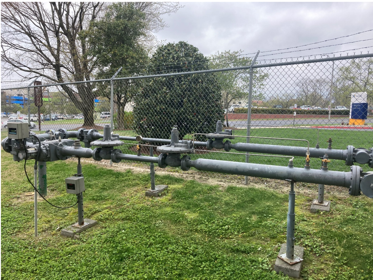
Natural Gas Monitoring Station – TidalHealth Peninsula Regional in Salisbury, MD
