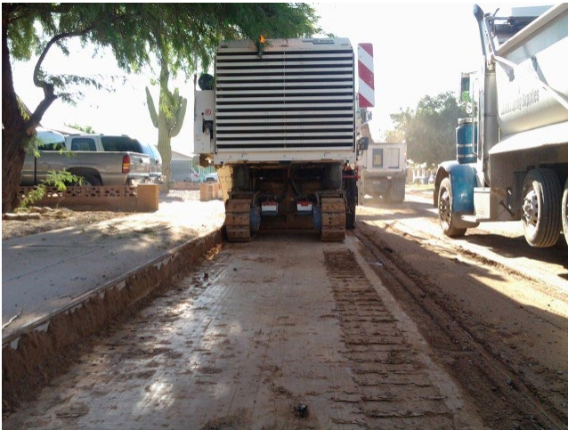
2. Typical asphalt pavement milling operation to remove the full depth of pavement.
