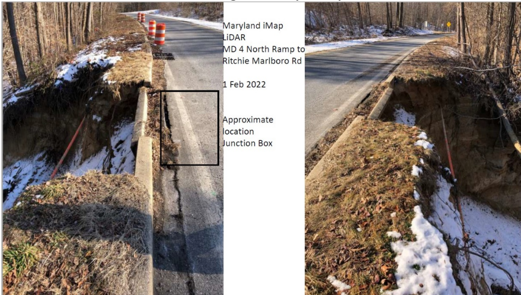
Image 1: Emergency design and repair- MD Route 4 Ramp to Ritchie-Marlboro Road Prince George's County, Maryland
