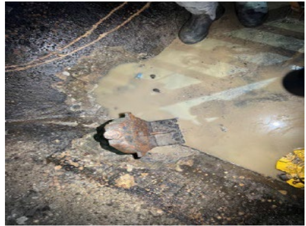
Water on bottom of tank a short time after it had been pumped dry
