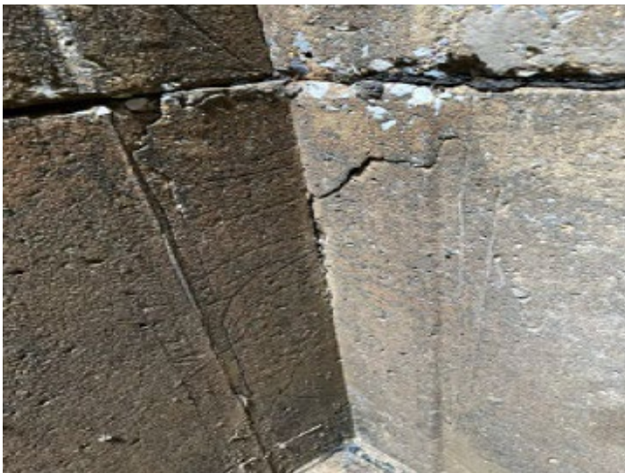
Cracks in Tank Wall
