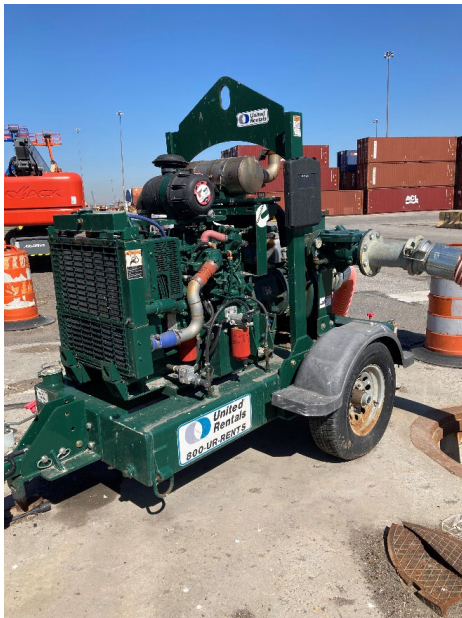
Figure 3 Pump at DMT
