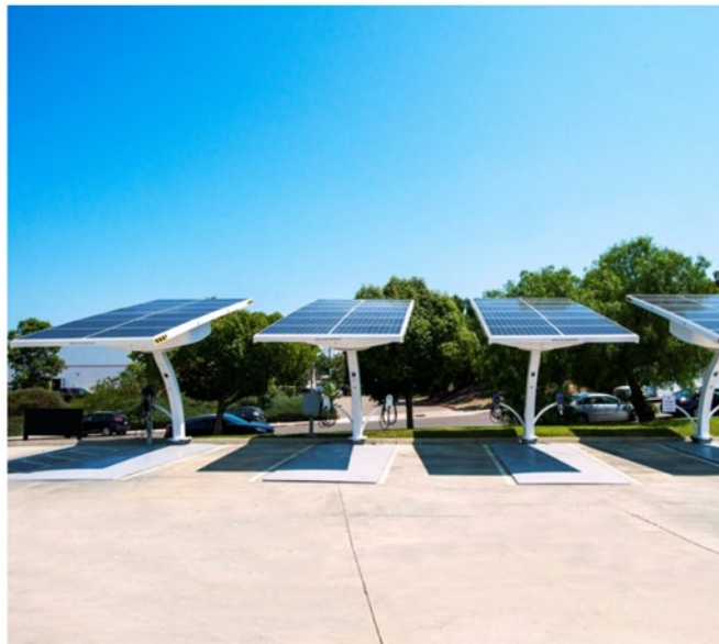
Figure 6 –Solar Based EV Charging Stations (courtesy of BEAM Global Inc.)
