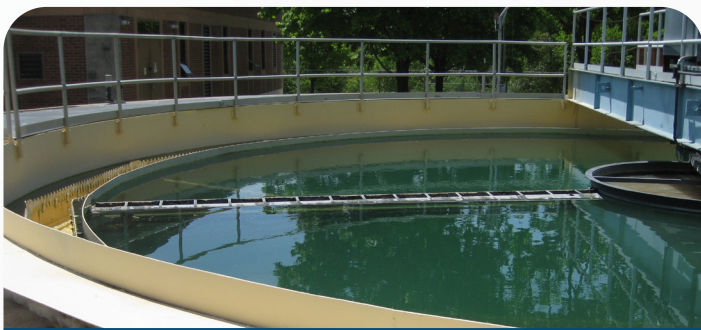
Dorsey Road Advanced Water/Wastewater Treatment Plant
