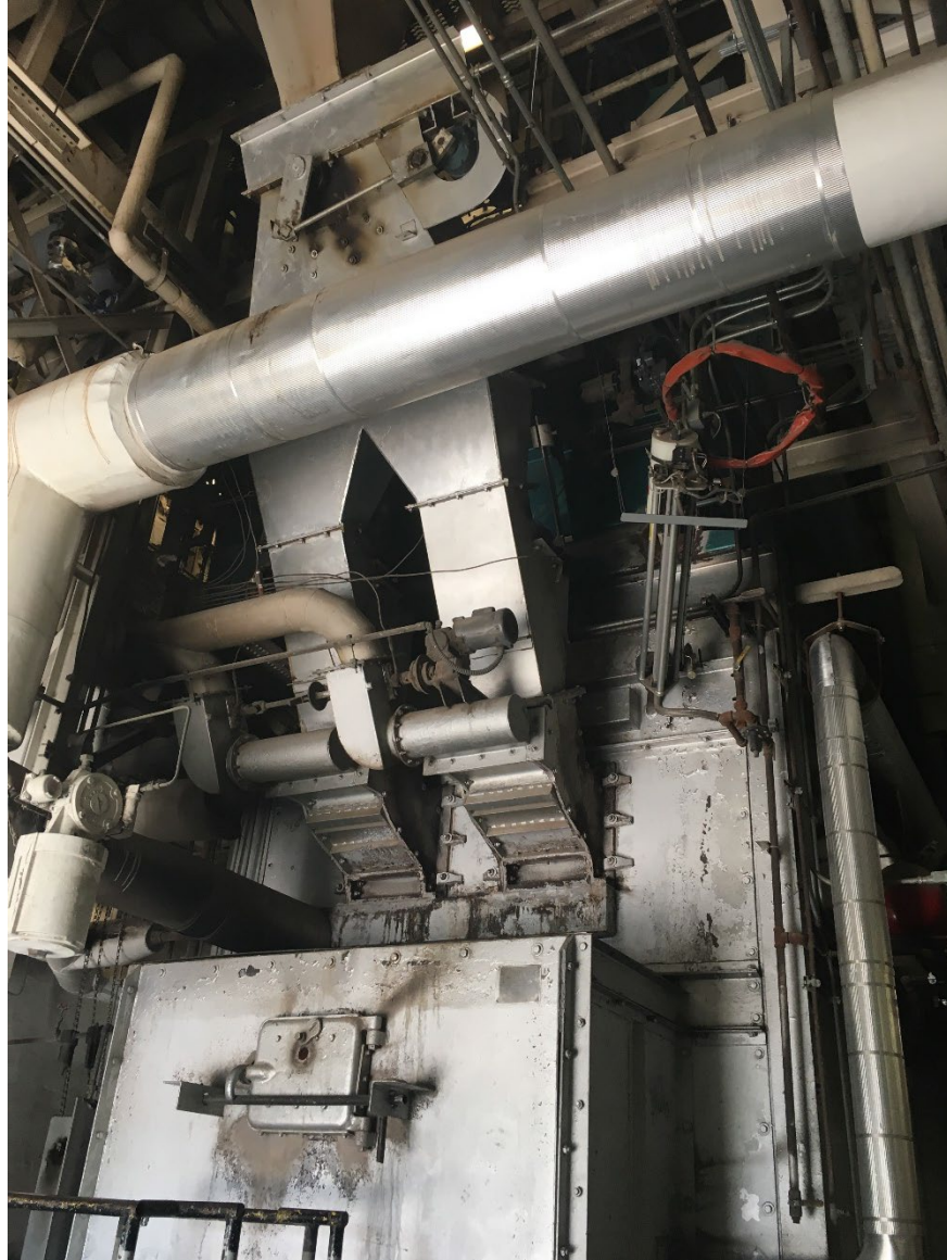
Boiler #2 at ECI Cogeneration Plant (view from front – shows firebox and wood chutes)
