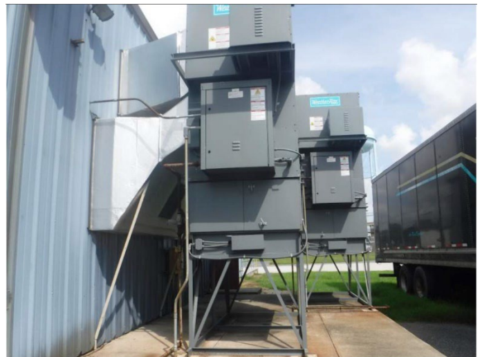
Existing outdoor equipment – MCE West
