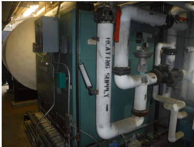
Existing indoor equipment – ECI Annex Worcester, Wicomico, and Somerset
