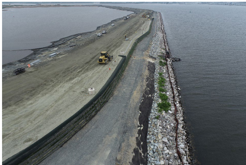
MSE wall being installed at Masonville DMCF as part of the Dike Raising to +30 Construction
