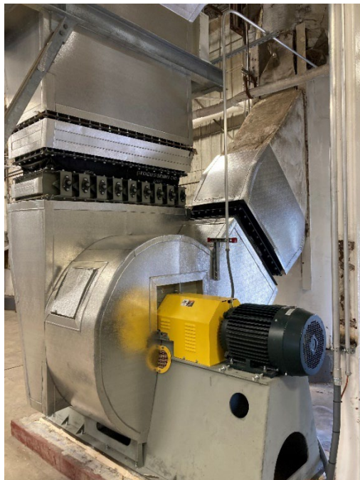
ID Fan for Boiler #2
