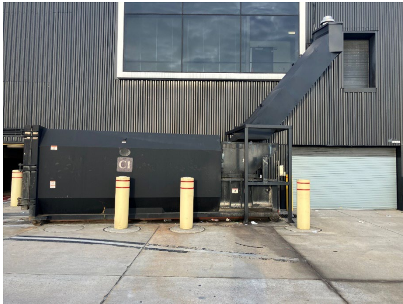
Figure 2- Airfield Trash Compactor C-1 with attached trash shoot
