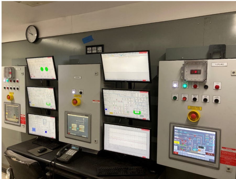
Boiler control system
