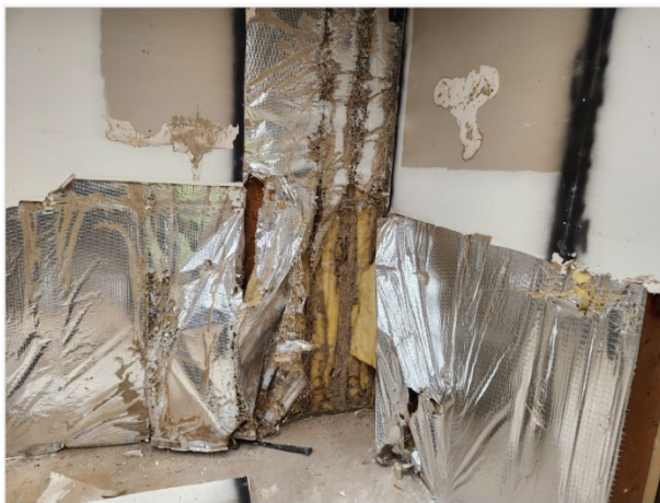
Scalehouse termite damage picture
