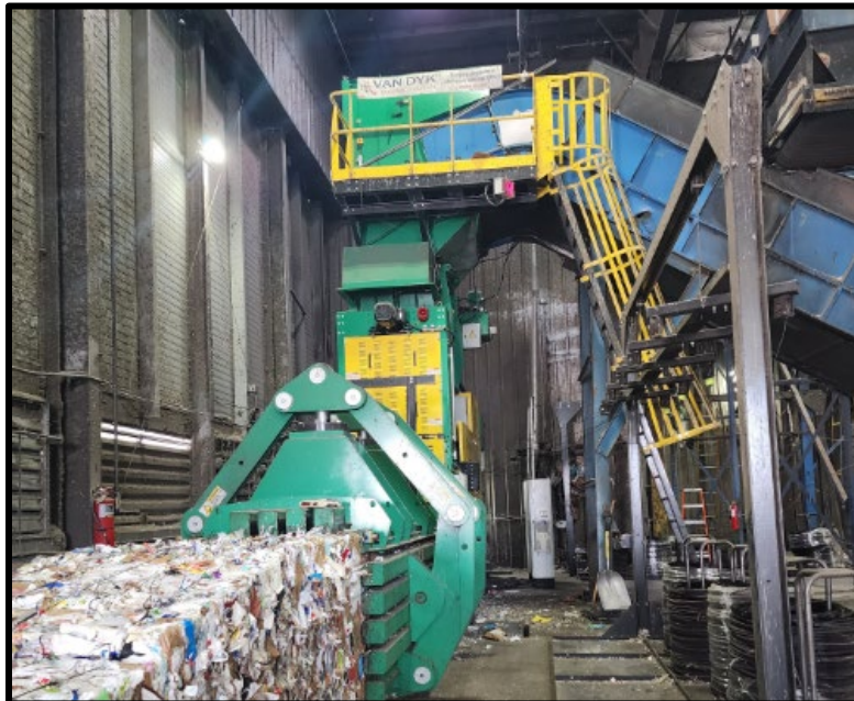
Prince George's County MRF – Inclined conveyor feeds into baler
