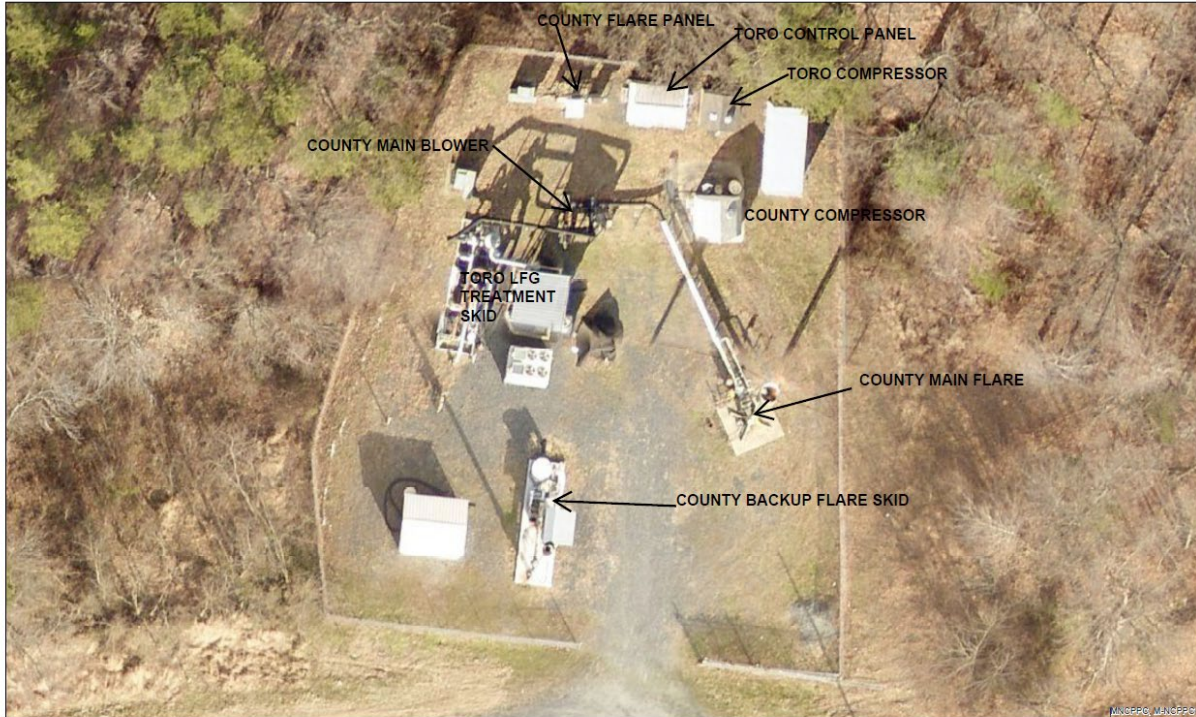
SANDY HILL CREATIVE DISPOSAL PROJECT - BLOWER FLARE STATION
