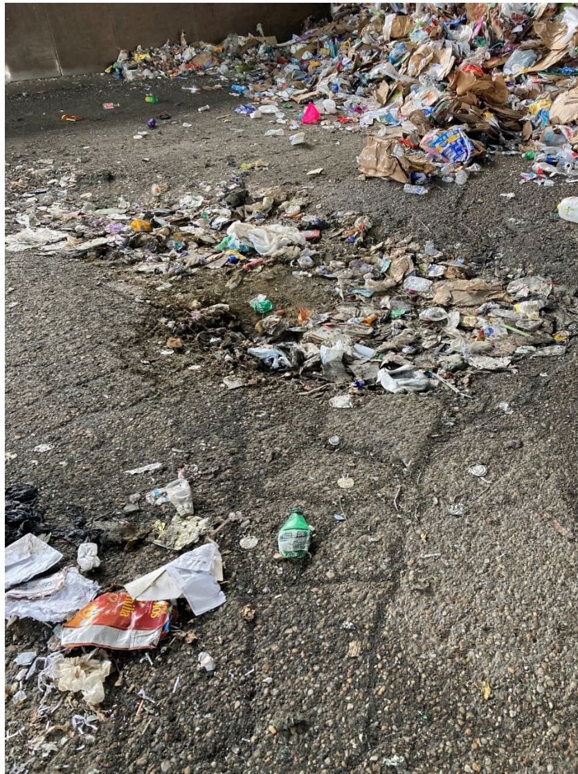
Tipping floor – Area Needing New Flooring Section
