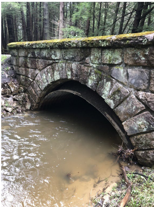
Collapsed Bridge culvert
