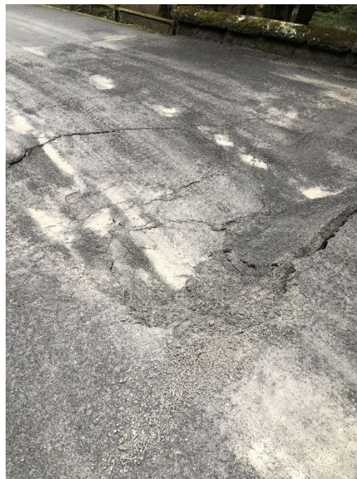
Sunken Pavement above culvert
