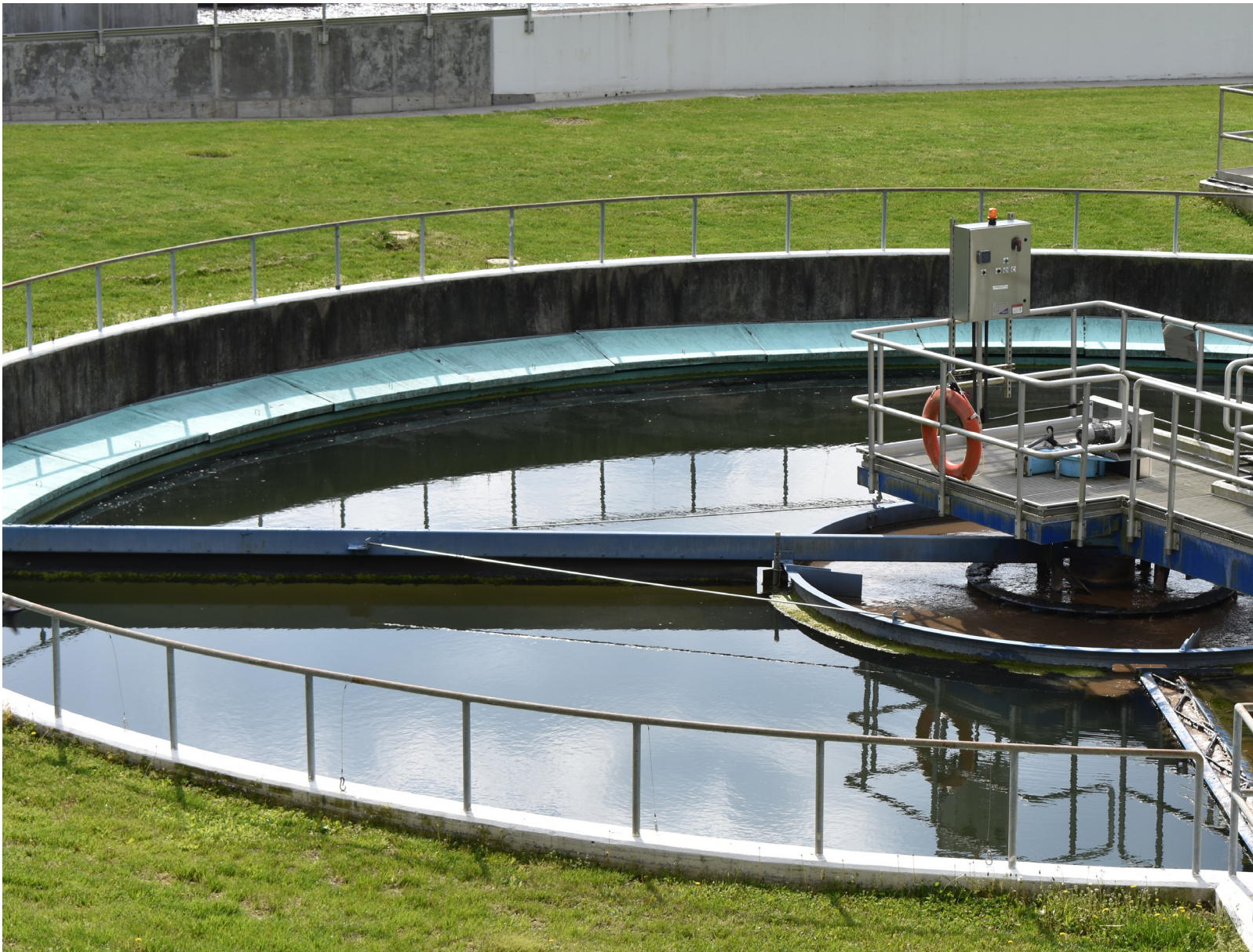
Freedom Wastewater Treatment Facility
