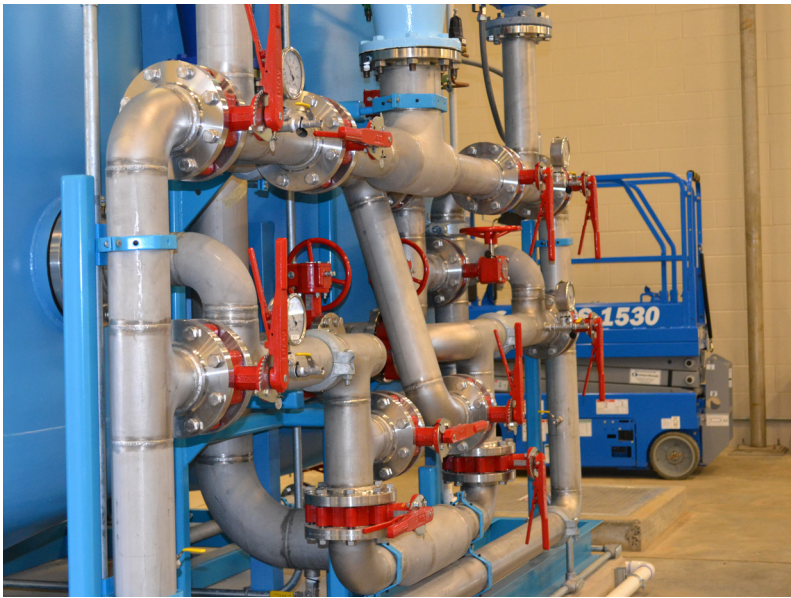
Rocky Gap Water Treatment Facility
